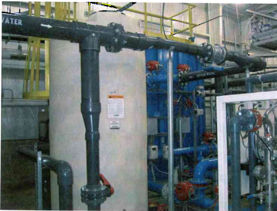
Figure 4.1 View of Influent line to Filters
